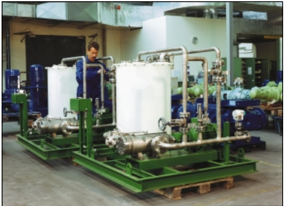
Tritec pumps on water injection skids
