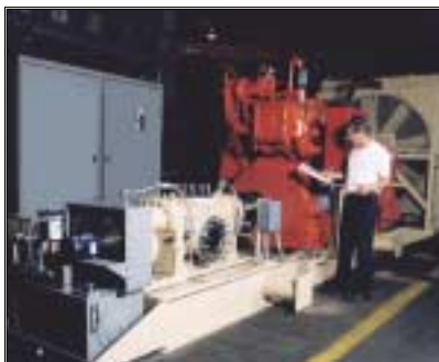
Typical crude oil pipeline pump with natural gas engine drive.
